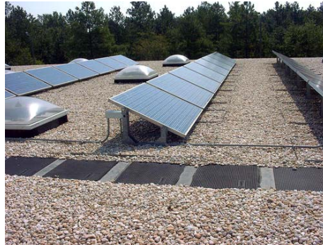
Figure C.13: Flat Panels Tilted on Commercial Building
