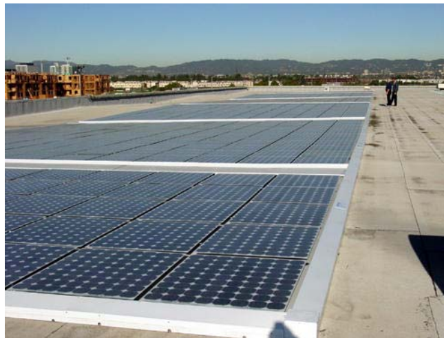
Figure C.14: Flat Panels Installed on Commercial Building
